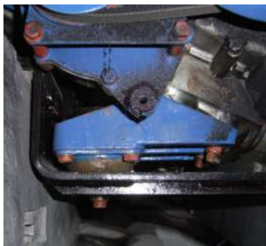
Front mounting viewed from under the engine facing aft and showing the mount sitting offset on the fabricated cross member.
