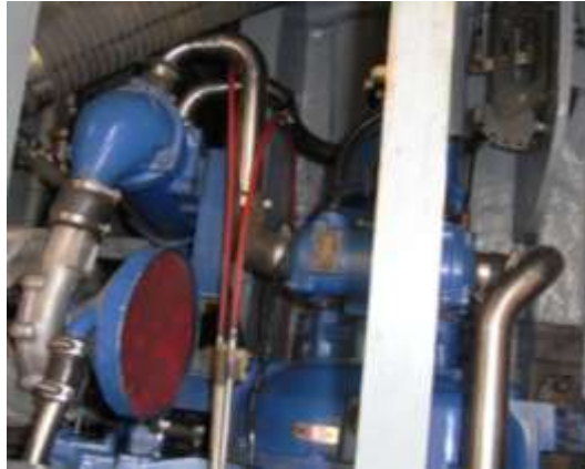
Raw water system fabricated from 1½” stainless tubing.
